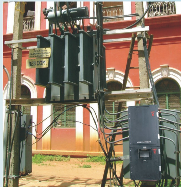
DTC Metering Box Serviced on pole
